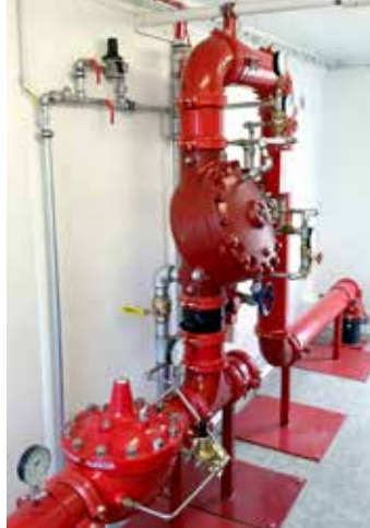
Sprinklerkerfi gastankur, pípulagningadeild.
